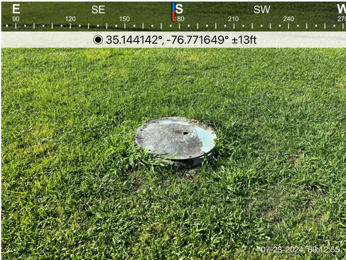
Photograph 5: Below grade vault with lid bolted shut in the northern portion of the site.
